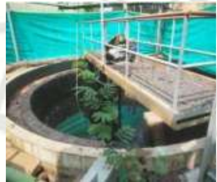
Photo 5: Clarifier filled with effluent in old ETP
