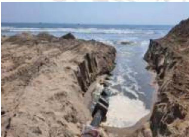
Photo14 : Effluent disposal on the shore through existing pipeline of 60m
