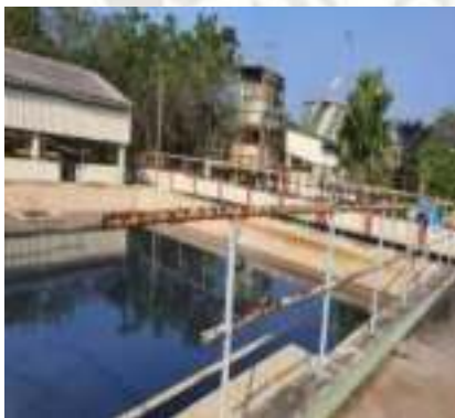
Photo 6: Effluent treatment plant
