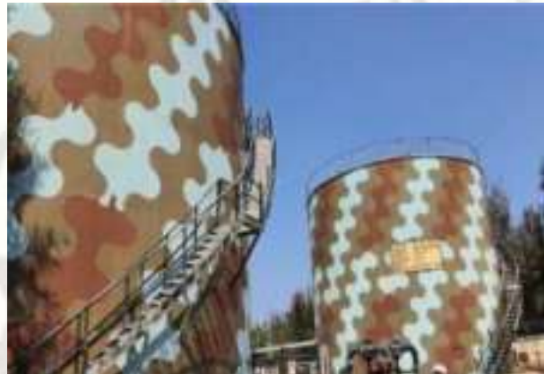
Photo13: new ETP treated effluent storage tank
