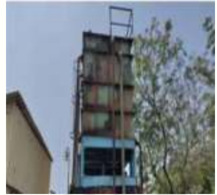
Photo 2: tilted plate interceptor
